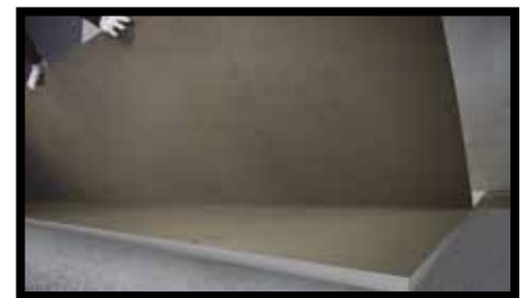
Fig.32 - Rest the slab on its long side and guide it down towards the floor.
